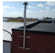
Roof mounted (n=461)
