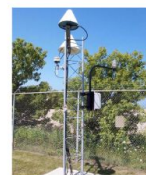
Steel tower (n=33)
